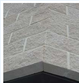
Split faced trough lintel blocks face and soffit (note: cut and bonded joint at 45° trough lintel block)
