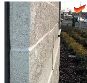
Good design detail. The split faced block has been ordered with one end shot blasted to add texture to the exposed end return into the window recess.
