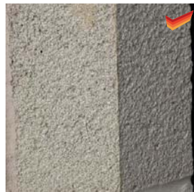
Good design detail. The block has been ordered with one face and one end shot blasted, to accommodate the exposed end in the recess.
