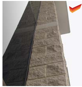
Good design detail. Shows full quoin block return into window recess. Block abutting window glass.
